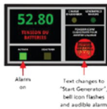
Figure: Battery Charge Drops to 55% or Less
