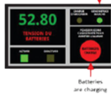
Figure: Generator Starts - Batteries are Charging
