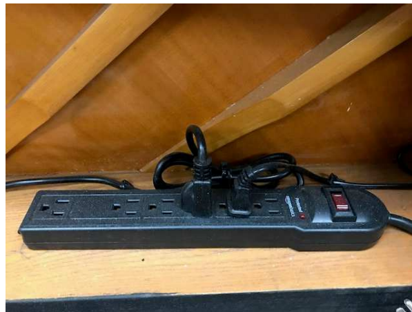
Illustration 139A – Power strip attached
