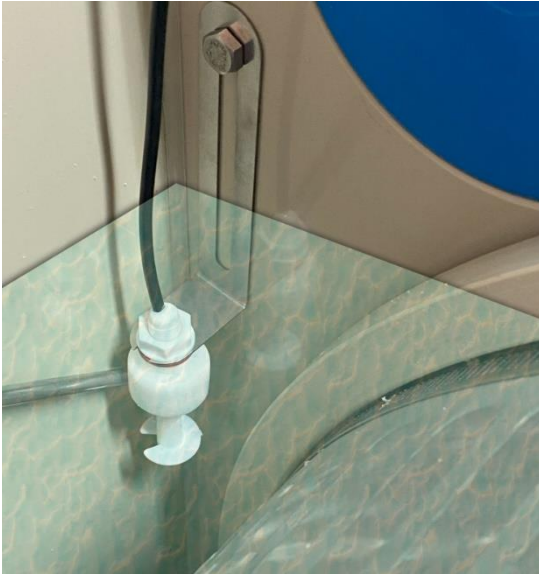
Float is in 'normal' position, pond pump is on.
