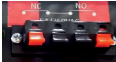
Remote alarm connection
