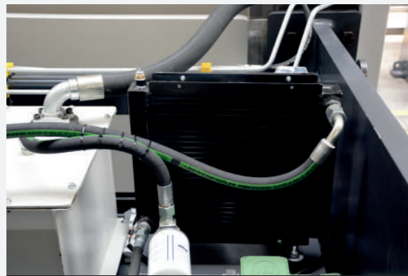
Hydraulic Oil Cooler System
