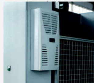
Electrical Cabinet Cooling System
