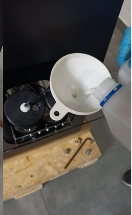
Figure 61. Filling the coolant tanks with distilled water
