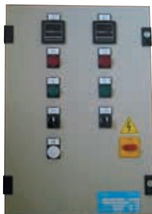
TWIN PUMP PANEL
