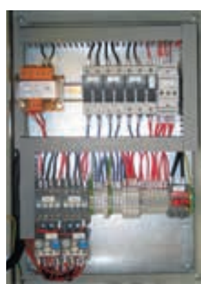
INTERNAL VIEW TWIN PUMP PANEL
