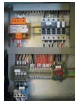
INTERNAL VIEW SINGLE PUMP PANEL
